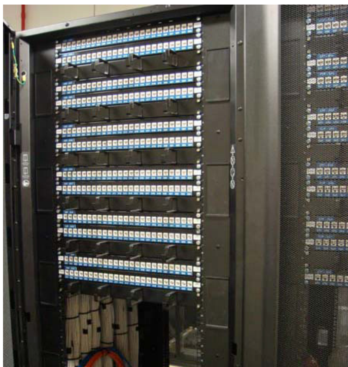
24-way patch panels and Traffolyte labelling system
