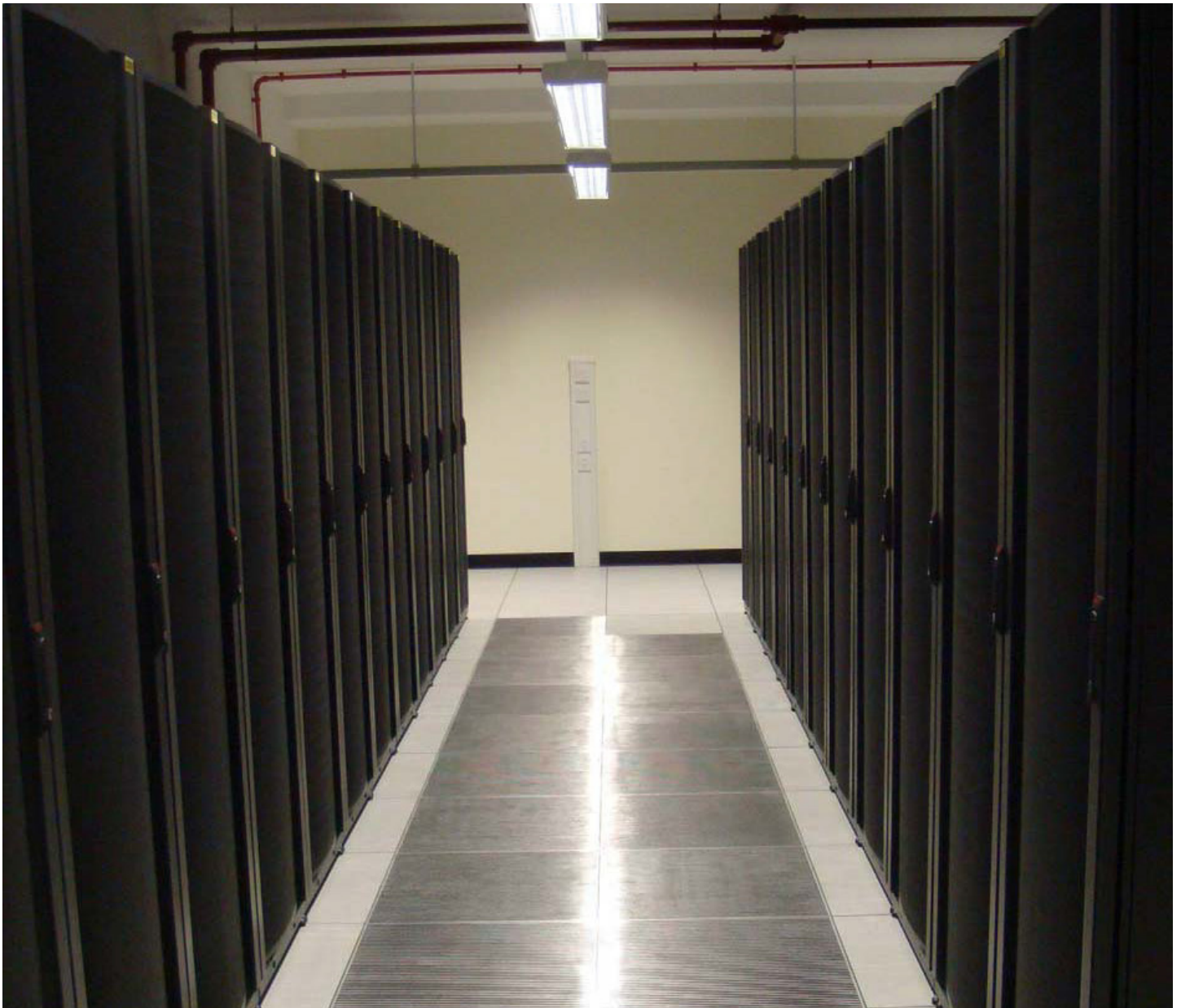
One of the cold aisles in this Tier 2 data centre. Connectix supplied over 3000 Category 6 pre-terminated cabling links also featuring a low flammability, zero halogen cable for higher fire protection.
