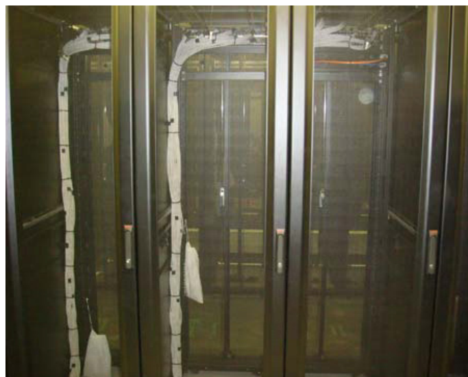
Each server rack was equipped with a 48-way Category 6 copper cable link going back to the main comm's row
